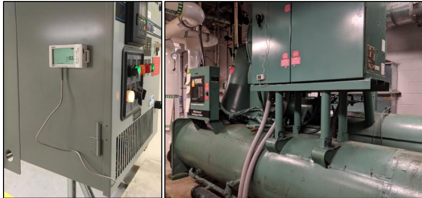
Figure 2. Current sensors installed on a single phase of a fan at Engineering Building-2 (left) and on a chiller at Toxicology Building (right) at NCSU.
